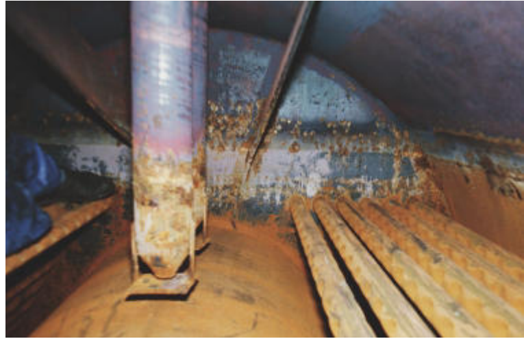
Shell boiler before the application of FINEAMIN®
