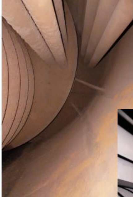
Shell boiler with deposits and corrosion
