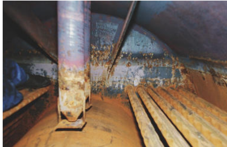
Boiler before the FINEAMIN® treatment
