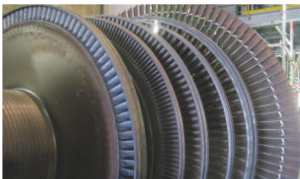
Steam turbine 29 MW
