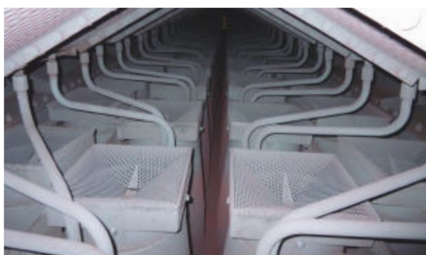
Steam drum boiler 98 bar
